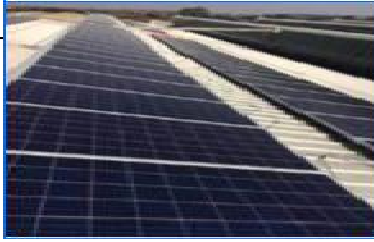
Roof top Solar panel
