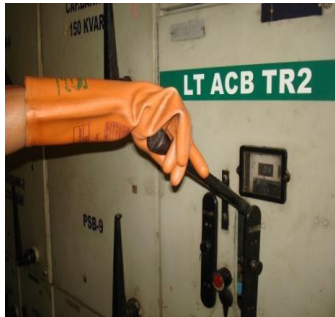
3. Air Circuit breaker for Protection.
